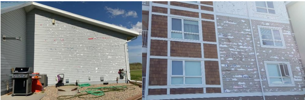
Figure 2. Severe vinyl siding damage (right-hand side wall only) (left) and contrasting damage to wooden and vinyl siding (right) on surfaces exposed to wind-driven hail.
